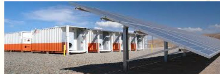
Solar panels and Battery rooms at Prosperity, PNM
